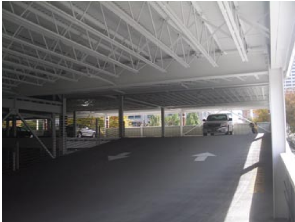
Throughout the garage, new joists were added in between the original joists to decrease the slab's span.
