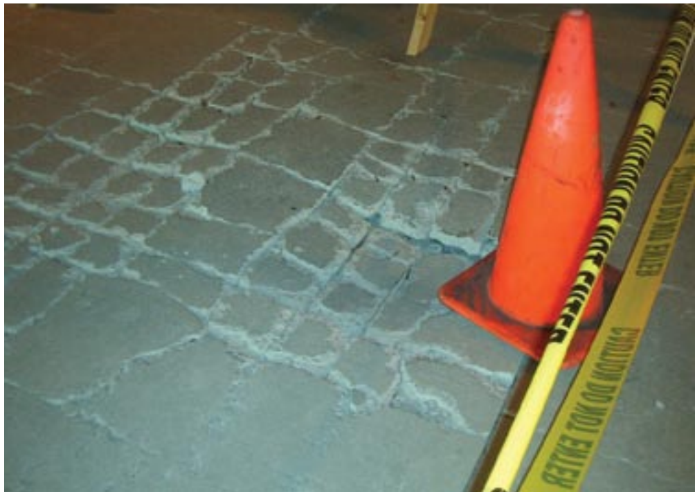
The original concrete slab was so badly cracked that it had punched through the deck in some places. Portions of the slab were barricaded.
