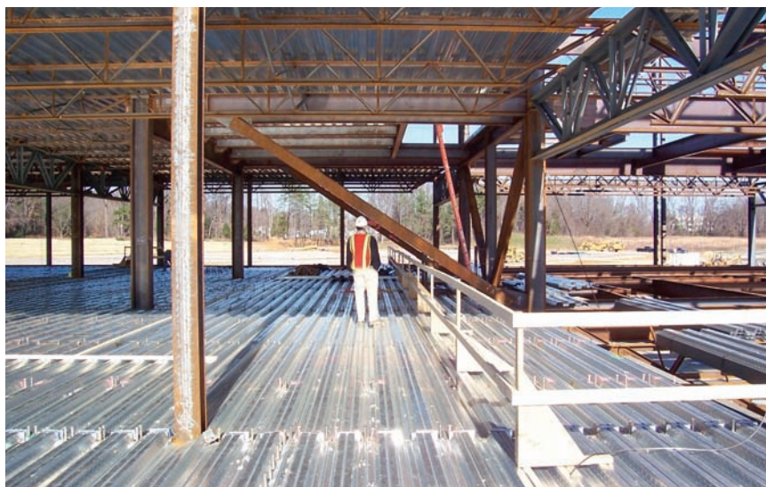
Composite steel joists with a depth of 44 inches, spacing of 9 feet, and span of 60 feet provide a very efficient floor system at Owens and Minor Inc., in Atlee Station, Va. A concrete slab having a total depth of 6 inches is supported by the 3-inch composite steel deck.
