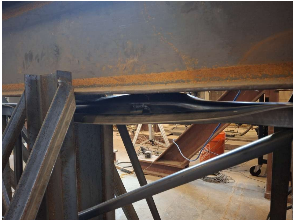
Figure 12. Failure mode for specimen F3a including twist of the top chord
