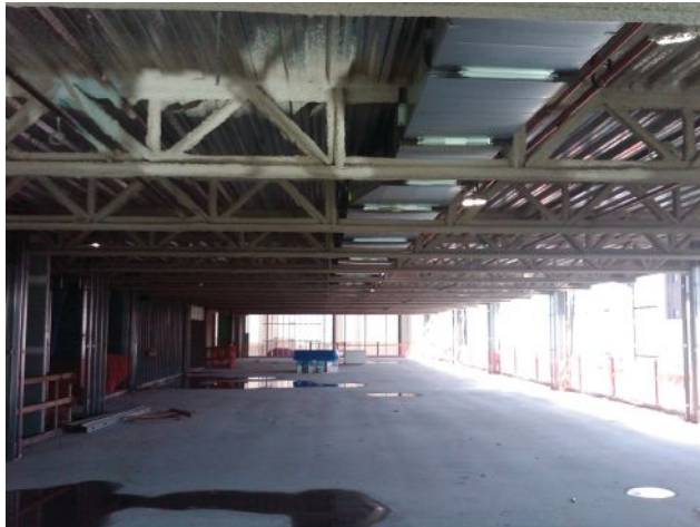
Figure 5. HVAC duct running through vierendeel opening.
