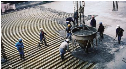
Figure 14. Concrete is placed over steel deck and supporting steel joists with a bucket.
