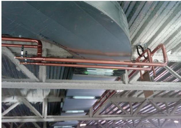
Figure 6. HVAC duct passing through vierendeel openings at the joist mid-span.
