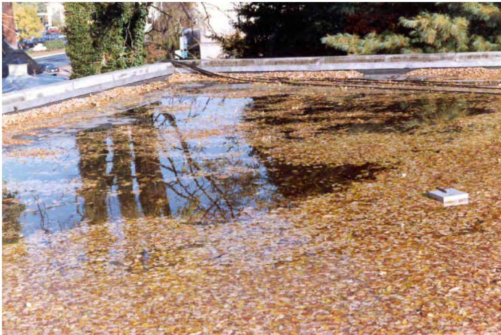
FIGURE 1.1 Potential for Roof Ponding Instability due to Blocked Drains (with permission from DEP Montgomery County, MD)
